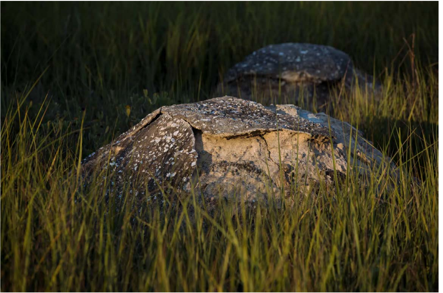
Seen up close, the “Marsh Ruins” reveal gaps in the tabby outer layer and fissures in the concrete substrate, the result of decades of exposure to the weather and the tide. Kendrick Brinson for The New York Times
